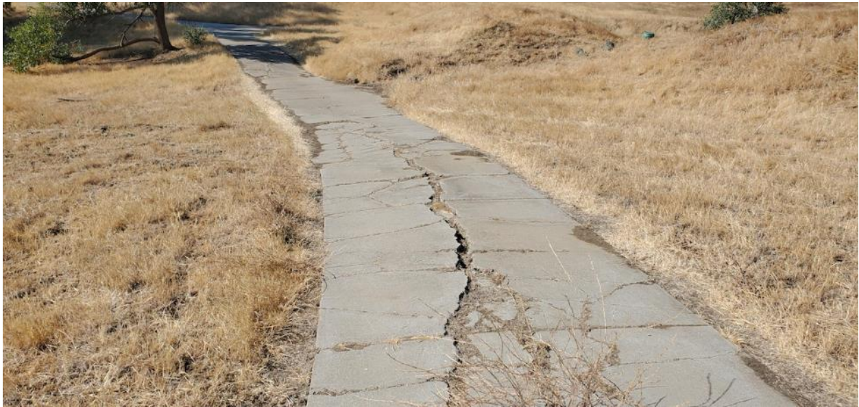
Photo 15. Concrete golf cart path with buckling concrete that may provide refugia for special status species. Facing south. July 16, 2020.
